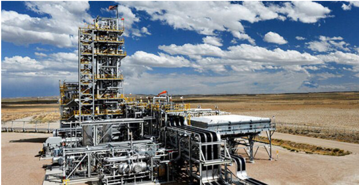
Shute Creek Treating Facility Source: ExxonMobil
