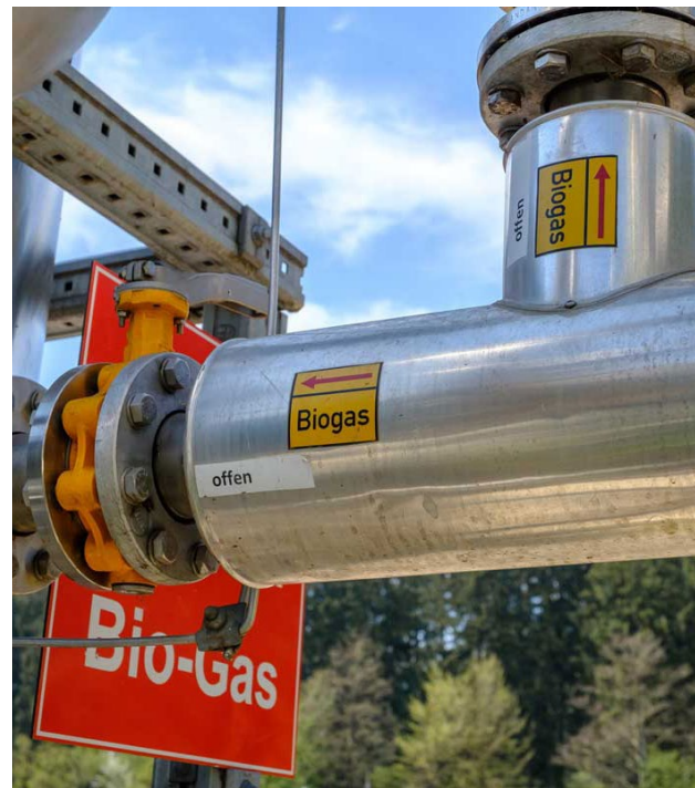
Biogas pipeline leading to the combined heat and power unit
