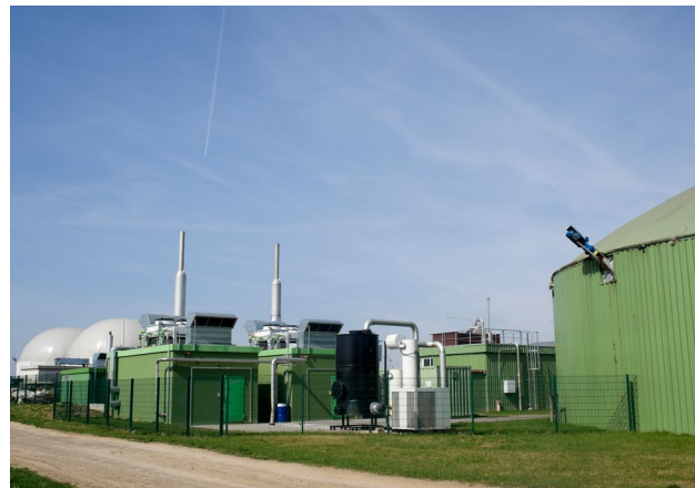
Two generators using biogas, and digesters
